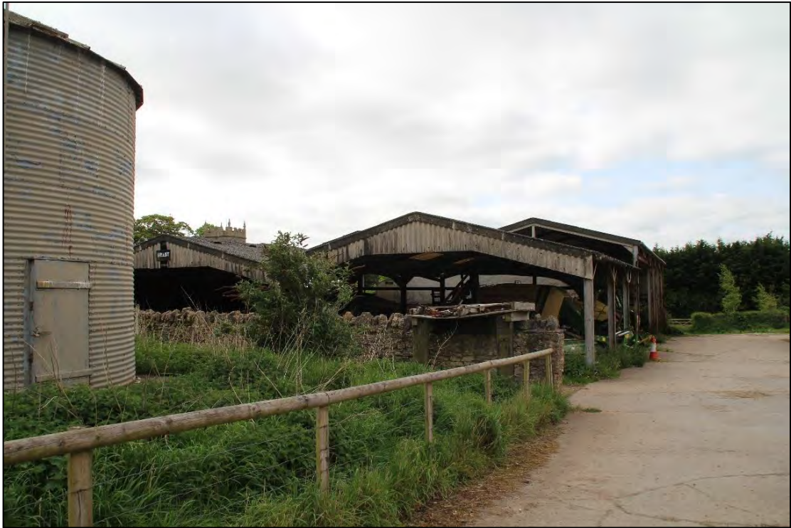
Photo 5 View of the sheds H and I from the north looking south with slurry tank in foreground
